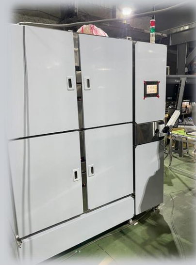
Tape storage equipment
